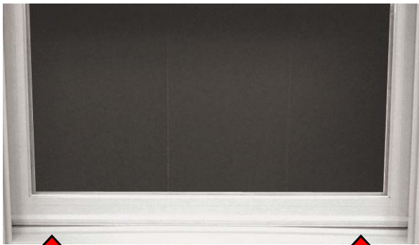
Inadequate Bulb Seal Compression
