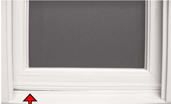
Inadequate Bulb Seal Compression
